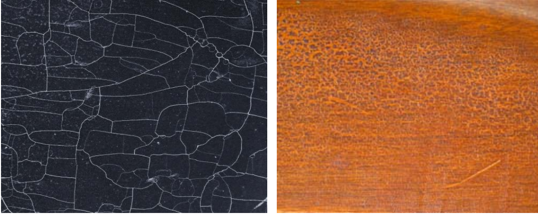
Crazing of finished surfaces
