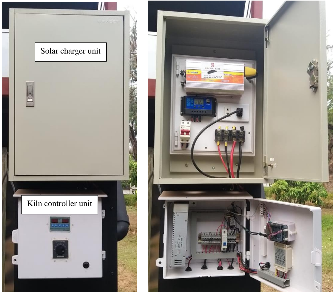
Figure 8. Solar charger and Kiln controller unit
